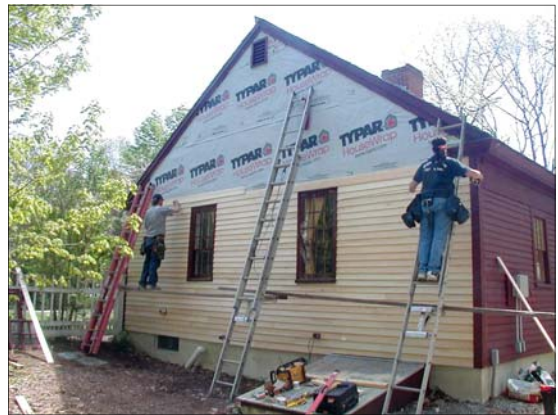
The Museum gets a new north wall and second story window (installed after this photo). Workers from DeHart Construction use historically correct custom-made clapboards.
