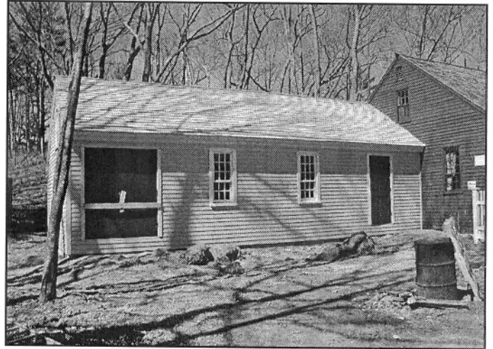
The new Winn House ell, showing the roof completed, the doors in place, and the shell essentially done.
